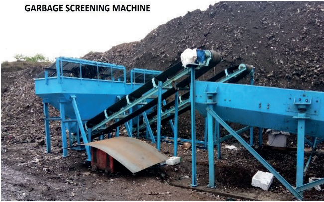
Figure 3: Garbage Screening Machine
