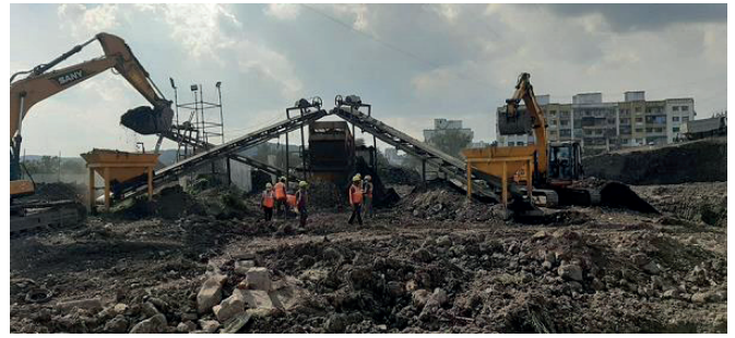
Figure 5: On Site Mass Screening Plant
