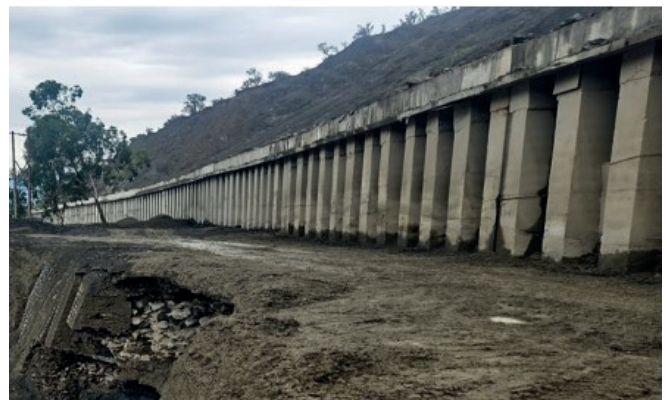
Figure 1: Typical Photograph of Slope Failure
