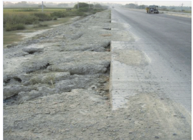
Photograph-1: Damage to Road Shoulders
