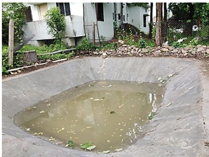
Coconut coir Cement Tank
