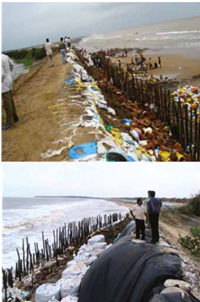
Photos-4 & 5: Coastal Erosion and Temporary Protection Measures at Pentha
