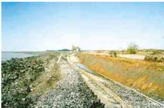
Damage to the railway line feeding Navalakhi port
