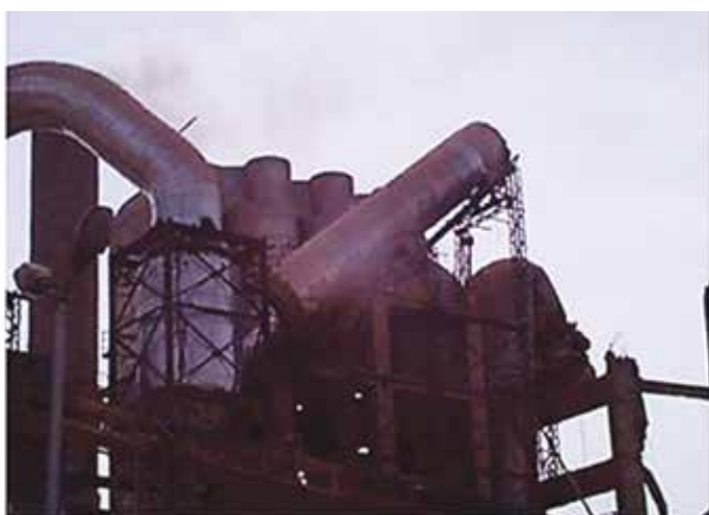
Damage at Sikka Cement Works
